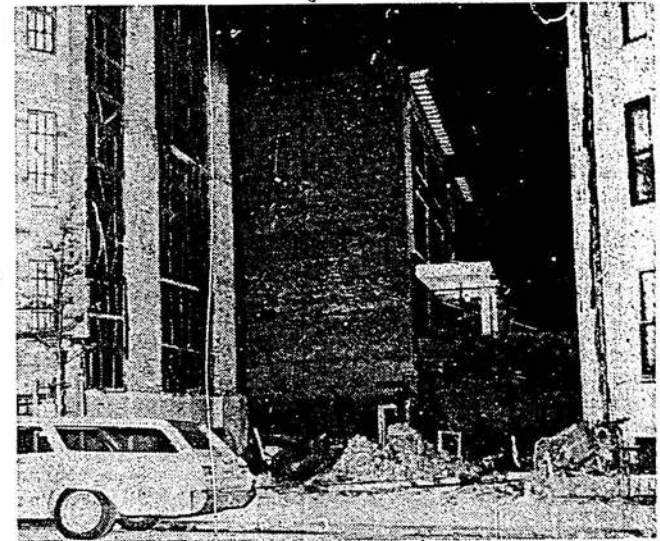
For the past few weeks demolition crews have entertained students gazing from the windows of Furst Hall by eradicating the two buildings that stood on the above spot. With hatchets and saws in their hands the workers reduced the structures to the present pile of rubble. When asked whether residents of the two neighboring buildings would be jeopardized by the crew's efforts, a University official replied, "that's their problem."
