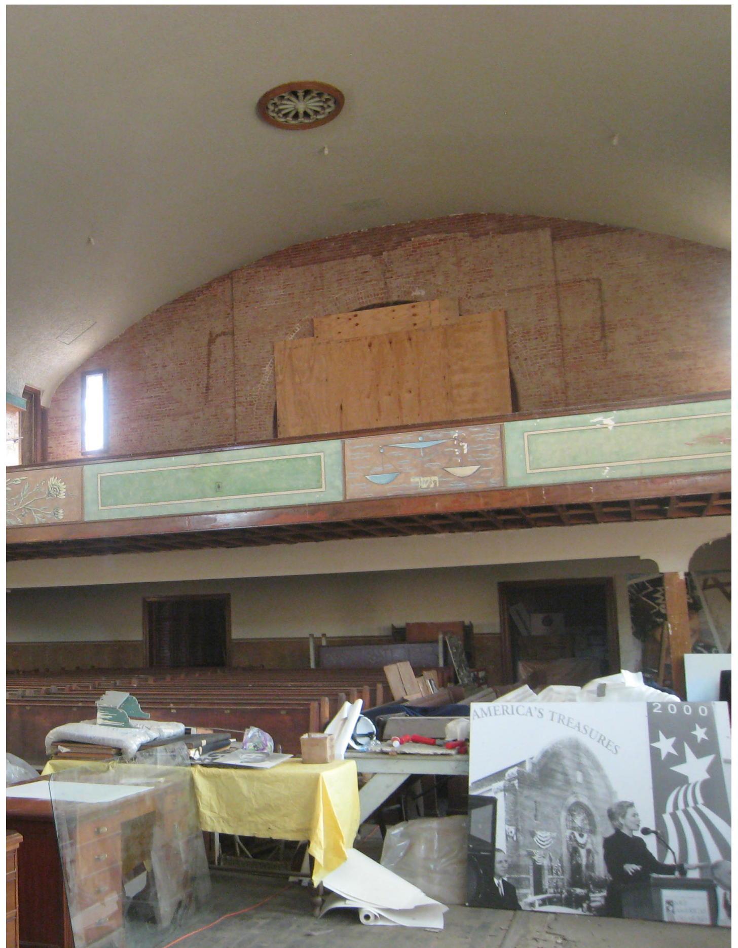
The Breed Street Shul in Los Angeles, California, which has deteriorated over time.
