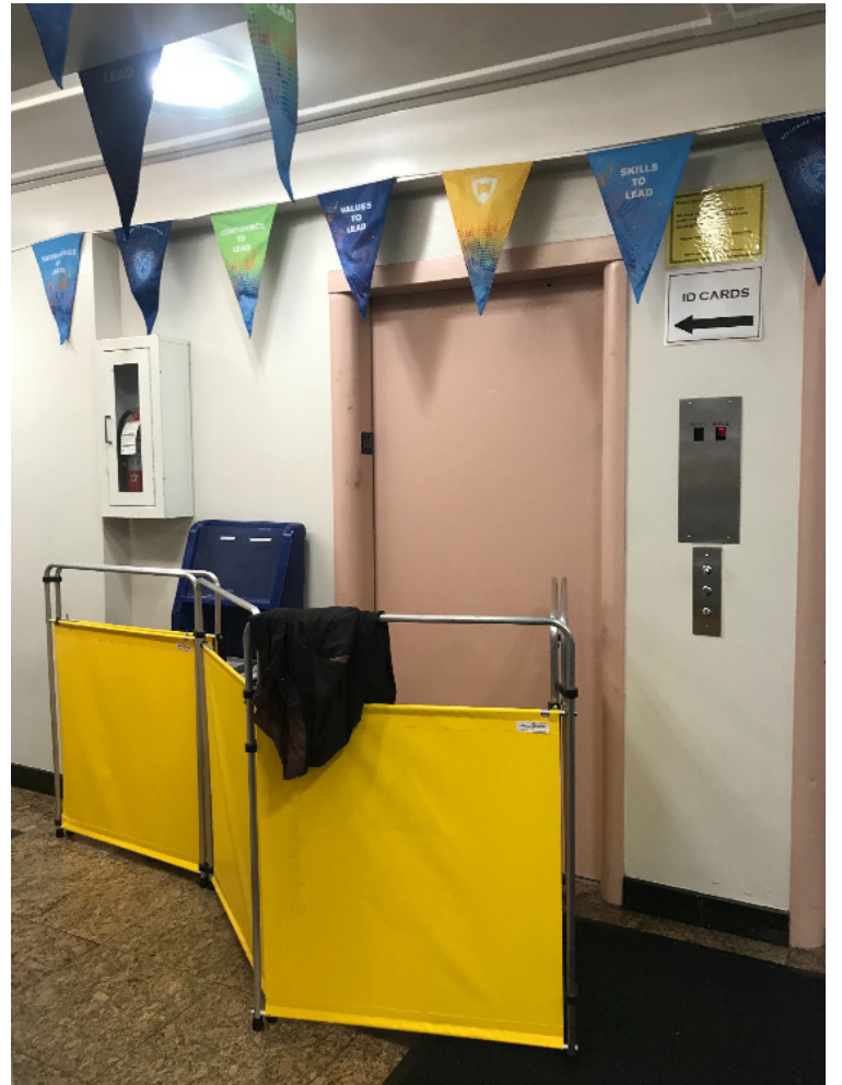
An out-of-service elevator
