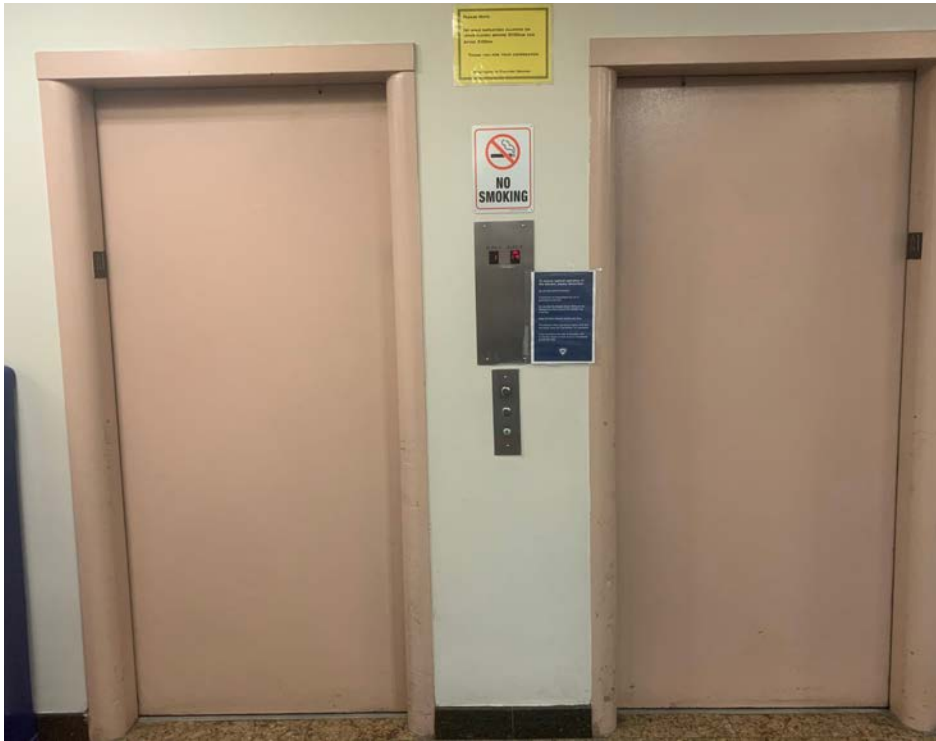
The Brookdale elevators are over 20 years old.
